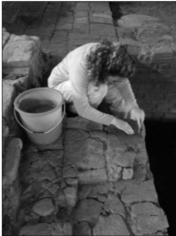
Figure 161. Plastering fissures and cracks
