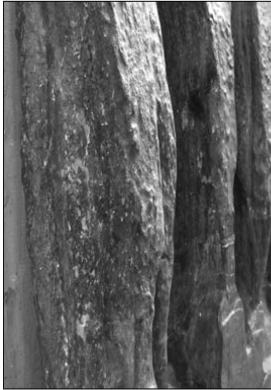
Figure 115. The hard resin caused scaling and stone powdering
