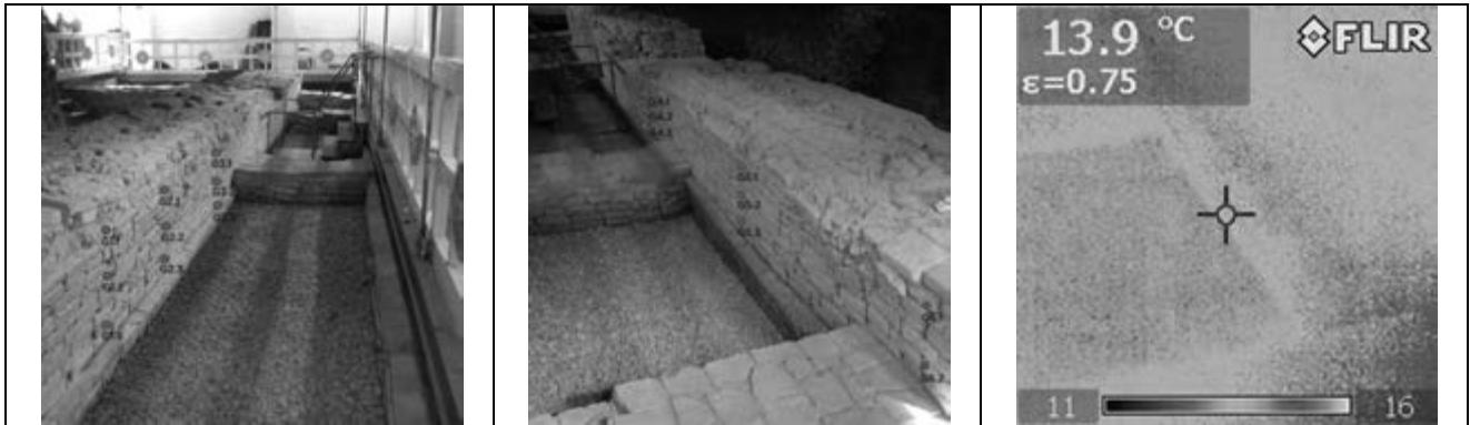
Figure 72. West Wall: Measuring point locations and water distribution of G4-G5-G6 locations.
