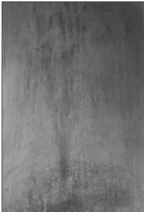
Figure 133. The corroded area on West side after the treatment with ESTEL 1000.
